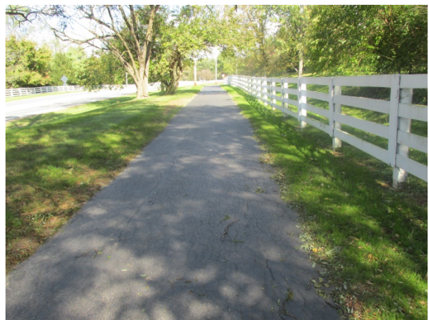
Cracks and deterioration at asphalt pavement walking path
