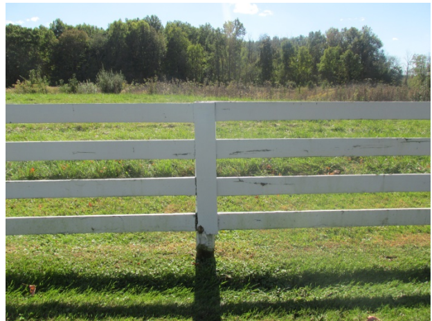
Wood deterioration at fence post
