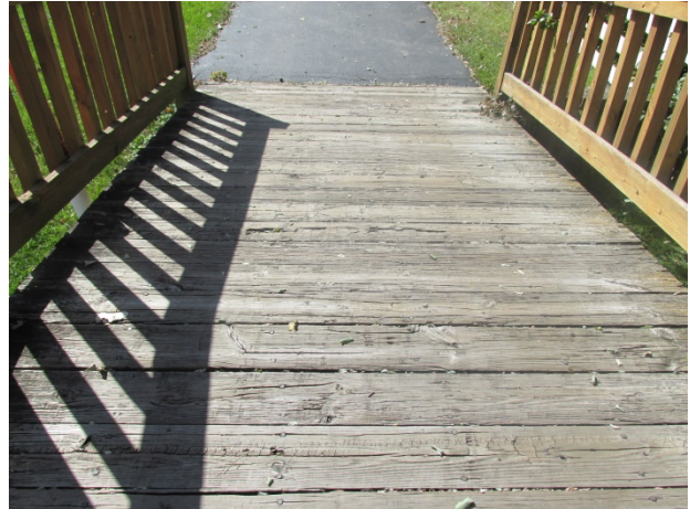
Worn deck boards at Route 62
