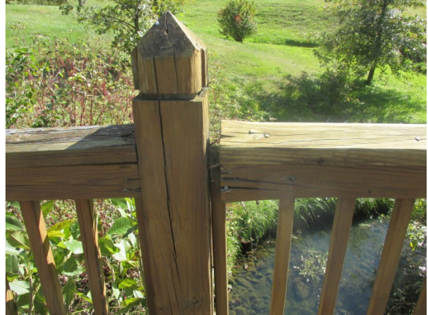
Detached railing at Route 62 Bridge
