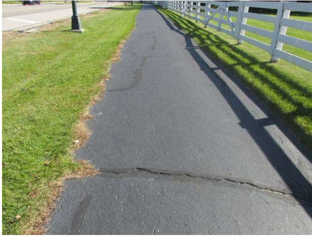
Cracks at asphalt pavement walking path
