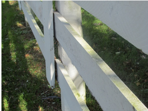
Loose connection at wood fence
