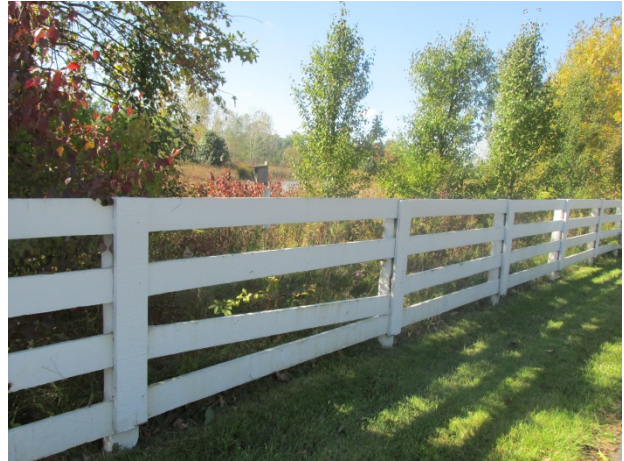
Loose rail at wood fence
