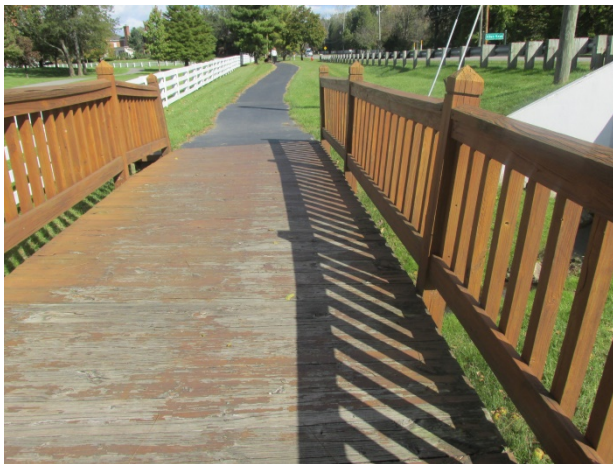
Bridge at Route 62 with worn deck board finish
