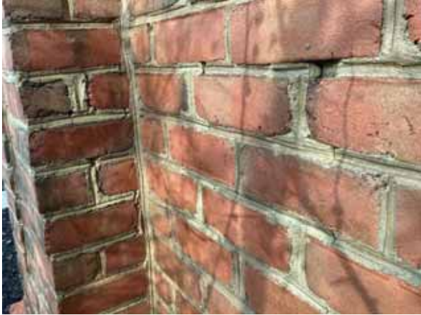
Mortar loss and evidence of previous repairs (New Albany Links Drive)
