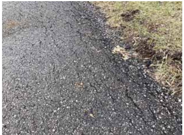
Pavement slippage at edge
