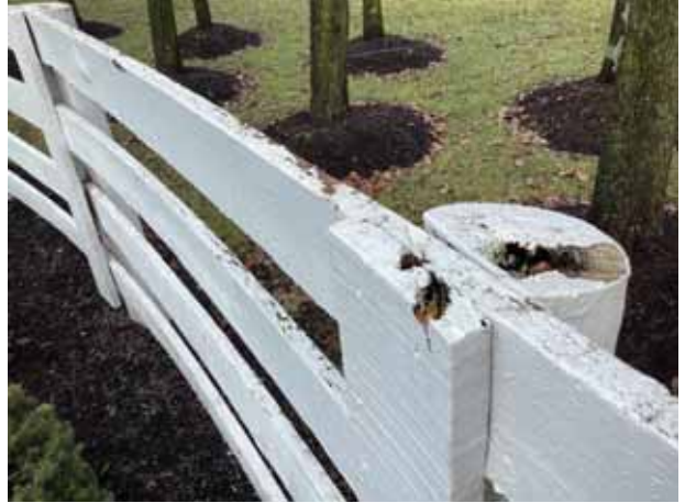
Wood rot and finish deterioration
