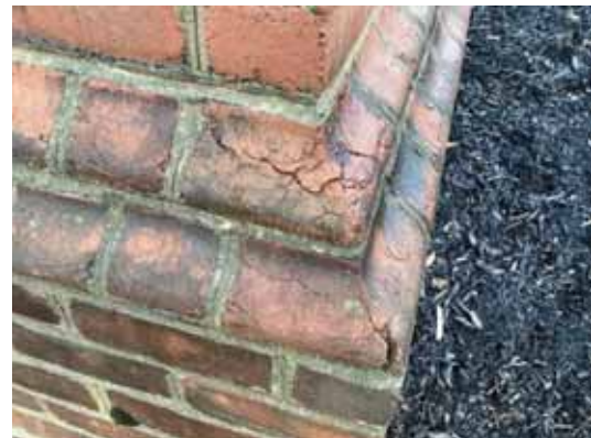
Masonry cracks and damage (New Albany Links Drive)
