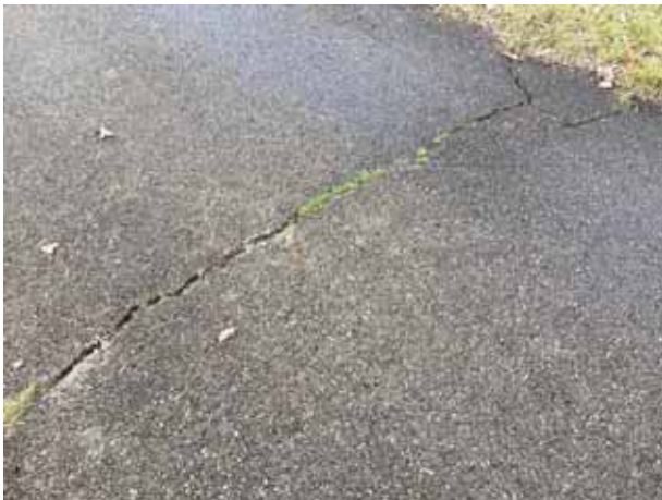
Pavement crack and organic growth
