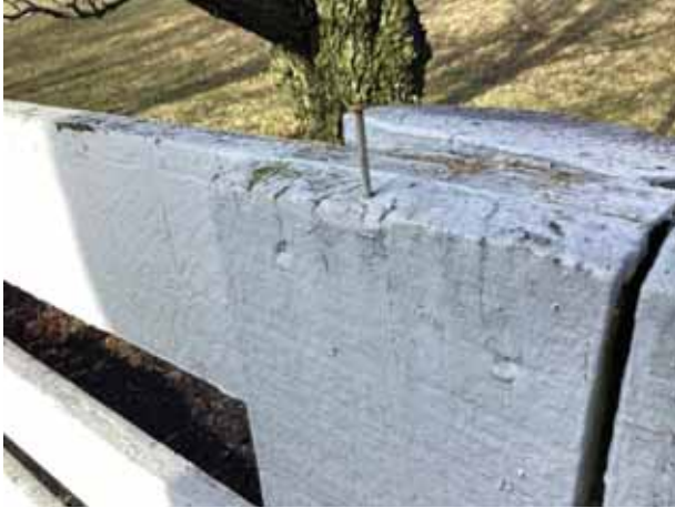
Popped nail and finish deterioration
