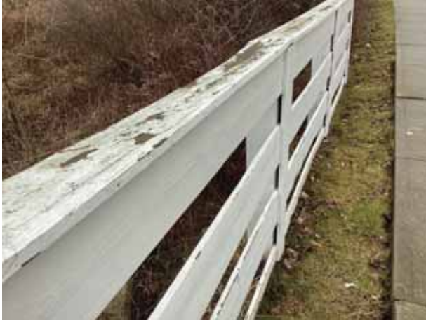
Deflection and finish deterioration
