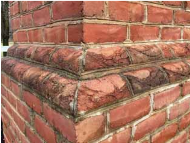
Masonry deterioration (Grate Park Drive)
