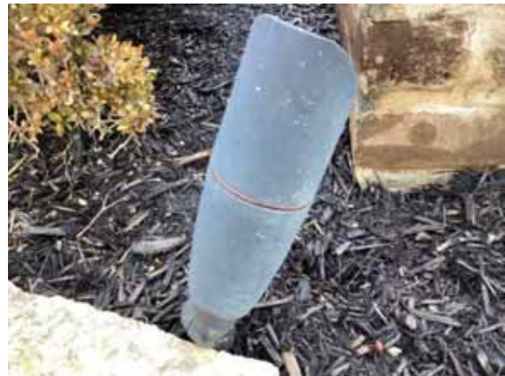
Light fixture – note finish deterioration (Skarlocken Green)
