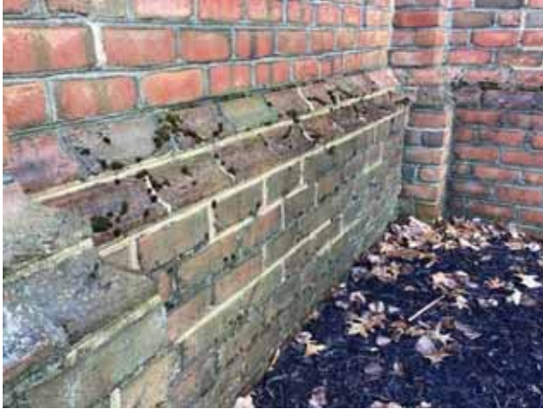
Organic growth and staining (Dean Farm Road)
