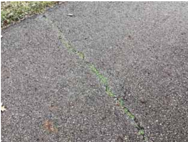
Pavement crack and organic growth
