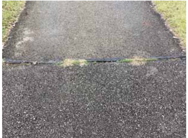
Organic growth at previous crack repair
