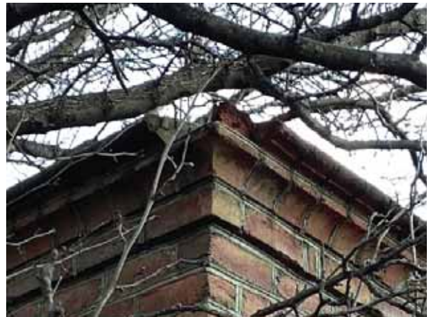
Masonry damage (Dean Farm Road)
