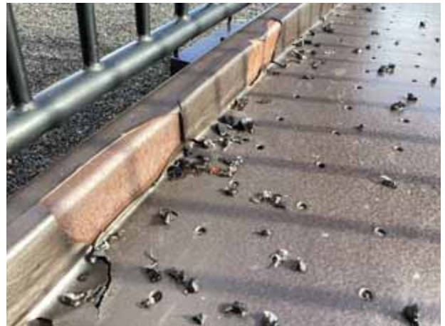
Peeling finishes and deterioration
