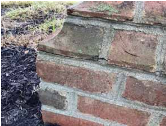
Mortar cracks (Skarlocken Green)
