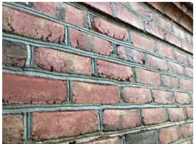
Masonry cracks (Dean Farm Road)
