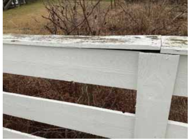
Deflection and finish deterioration
