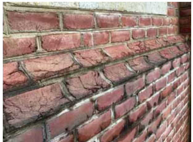
Masonry cracks and deterioration (New Albany Links Drive)
