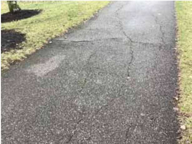
Pavement cracks and settlement
