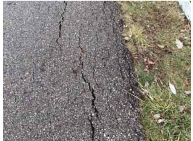
Pavement slippage at edge
