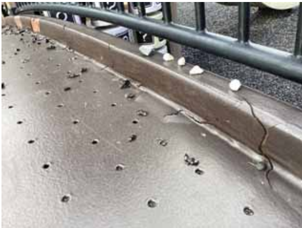
Cracks and deterioration
