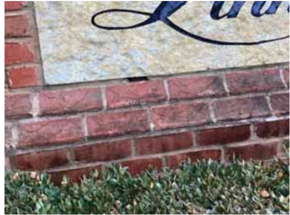
Mortar loss (Skarlocken Green)
