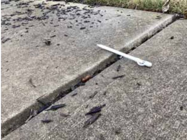
Trip hazard, shown at Skarlocken Green
