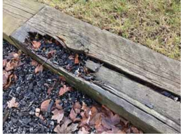
Wood rot at playground border
