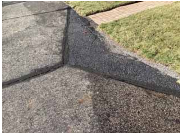
Previous patching and crack fill repairs
