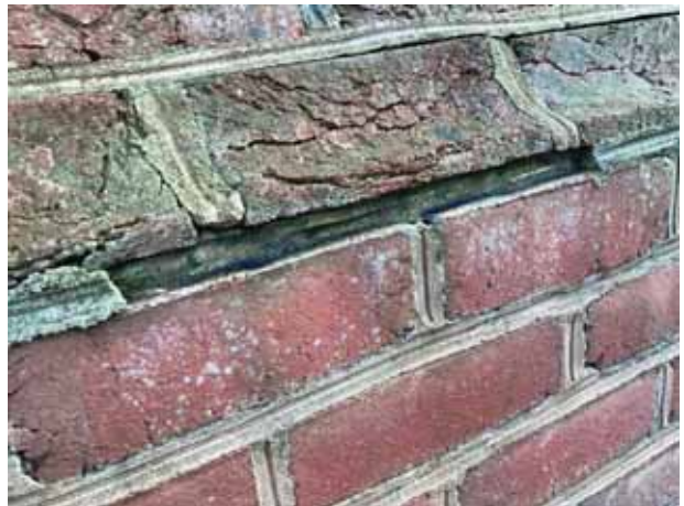
Mortar loss (New Albany Road East)
