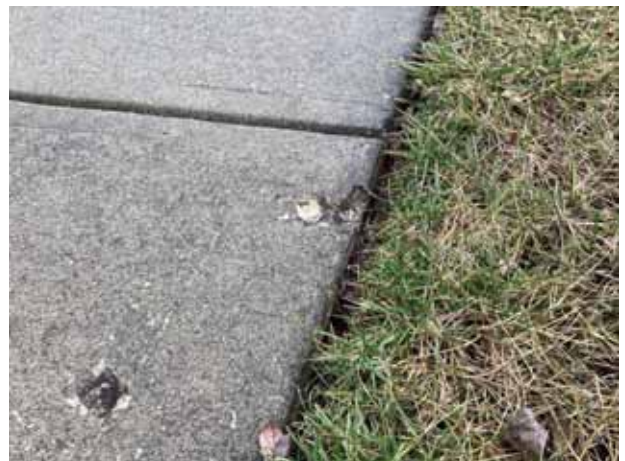
Minor concrete damage
