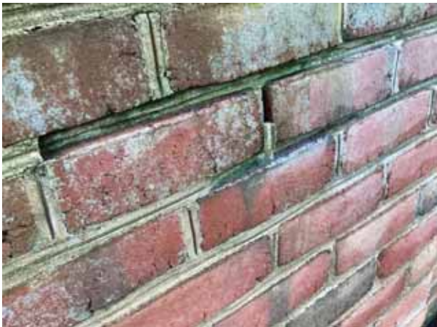
Mortar loss (New Albany Road East)
