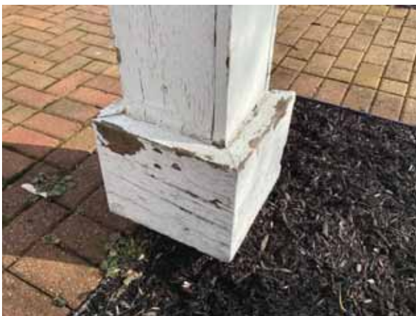
Finish cracks and deterioration
