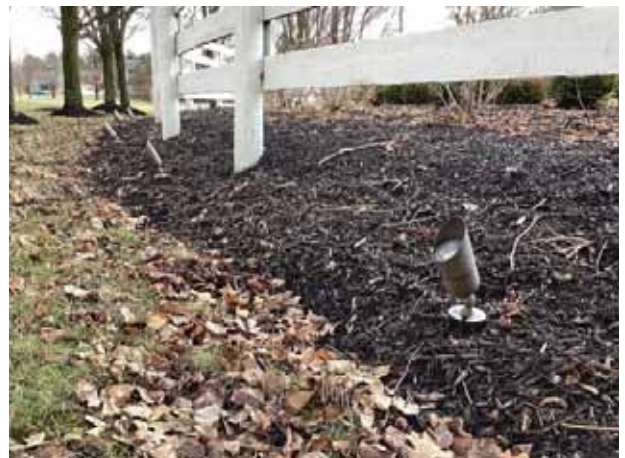
Lighting detail (Dean Farm Road)
