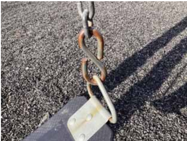
Rust and finish fade at swing
