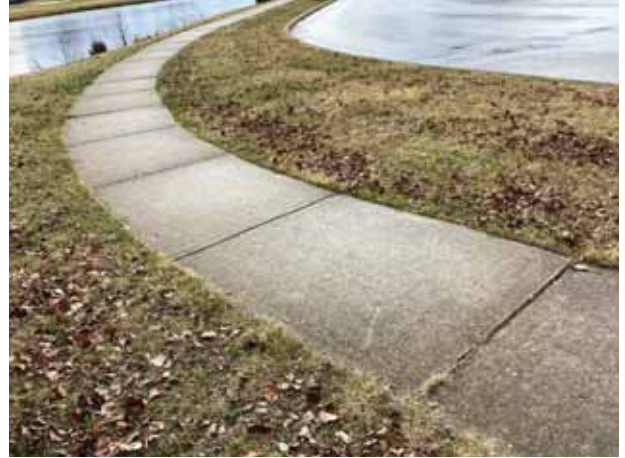
Concrete sidewalk overview – note minor settlement
