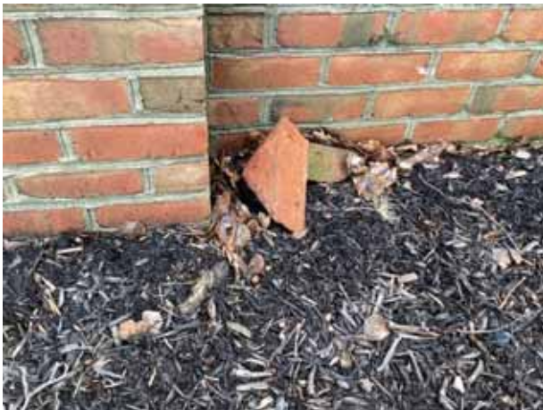
Detached masonry (Dean Farm Road)
