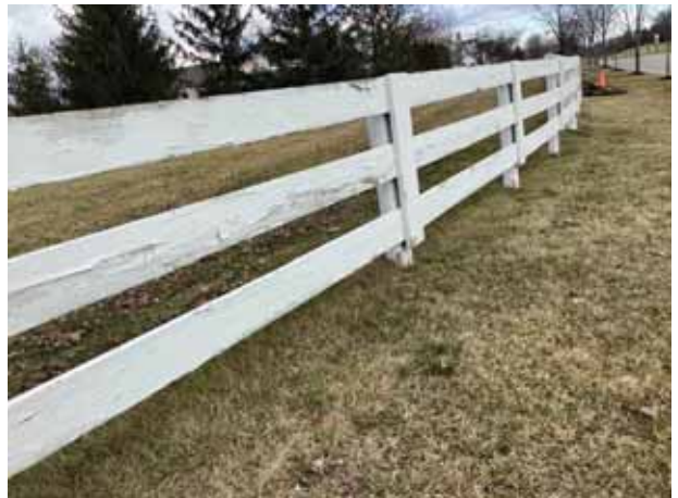
Peeling finishes and finish deterioration
