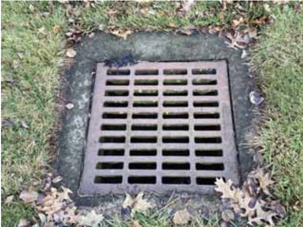
Landscape catch basin
