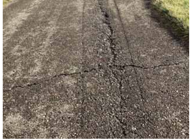
Pavement cracks and deterioration
