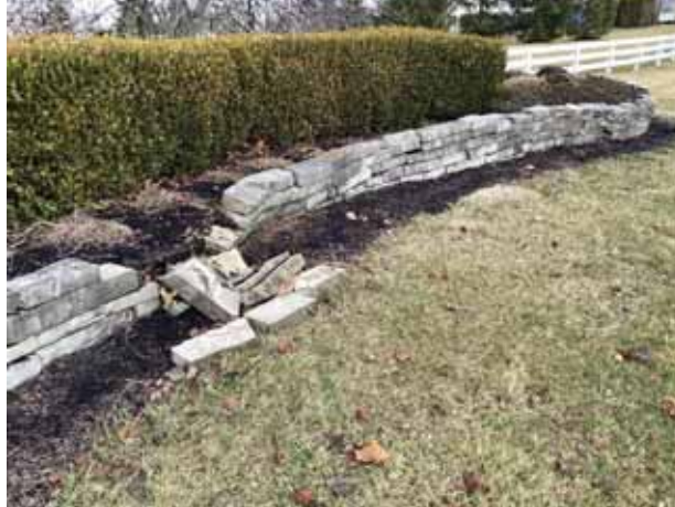
Stone retaining wall overview, note fallen stone
