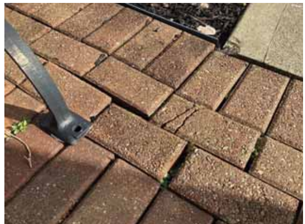
Settlement and damage
