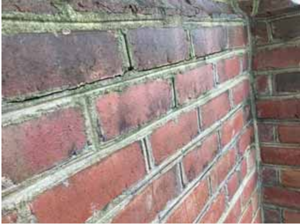
Mortar cracks (New Albany Links Drive)
