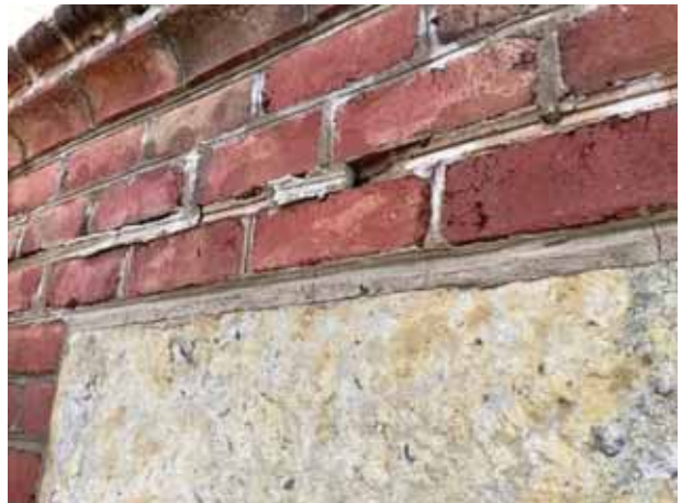
Mortar loss (New Albany Road East)
