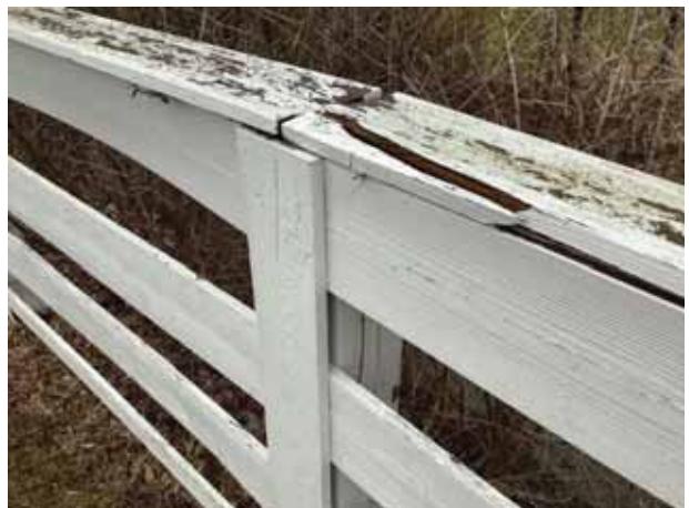
Wood rot and deterioration
