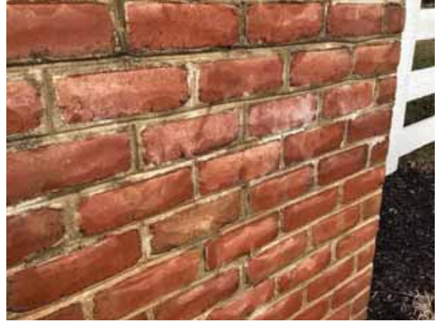
Efflorescence (Grate Park Drive)
